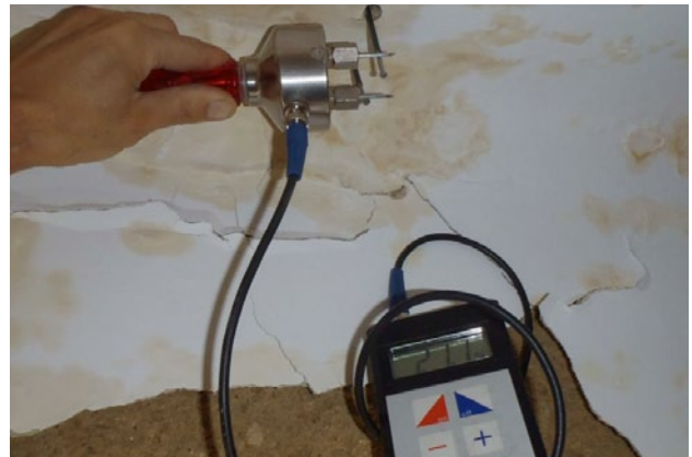
Figure 35. Measuring after water damage
